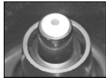
PB Fill connector 30 seconds after applying liquid leak detector.
